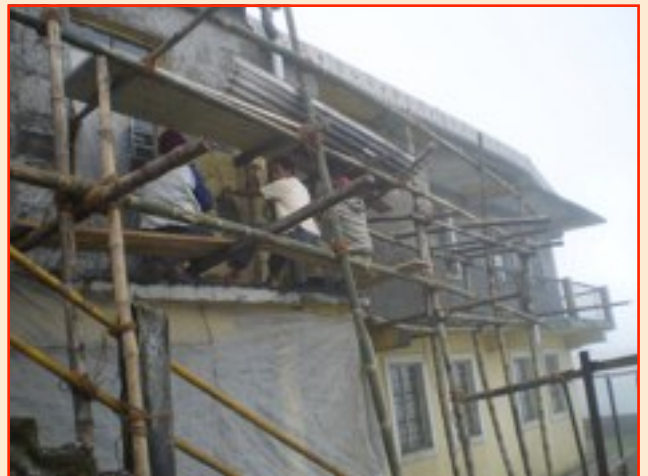
Rajesh & Niraj are repairing our backside building walls so they won't seep rainwater and let it inside.
